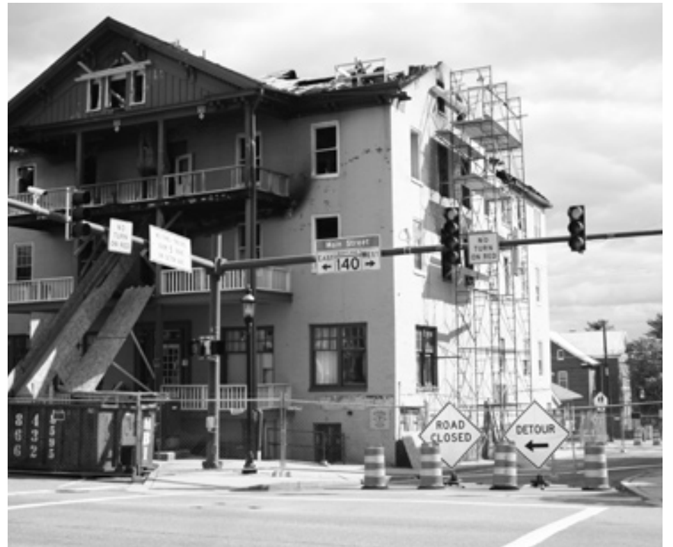
The Western Maryland Hotel under repair. See related stories on pages 21 and 29.
